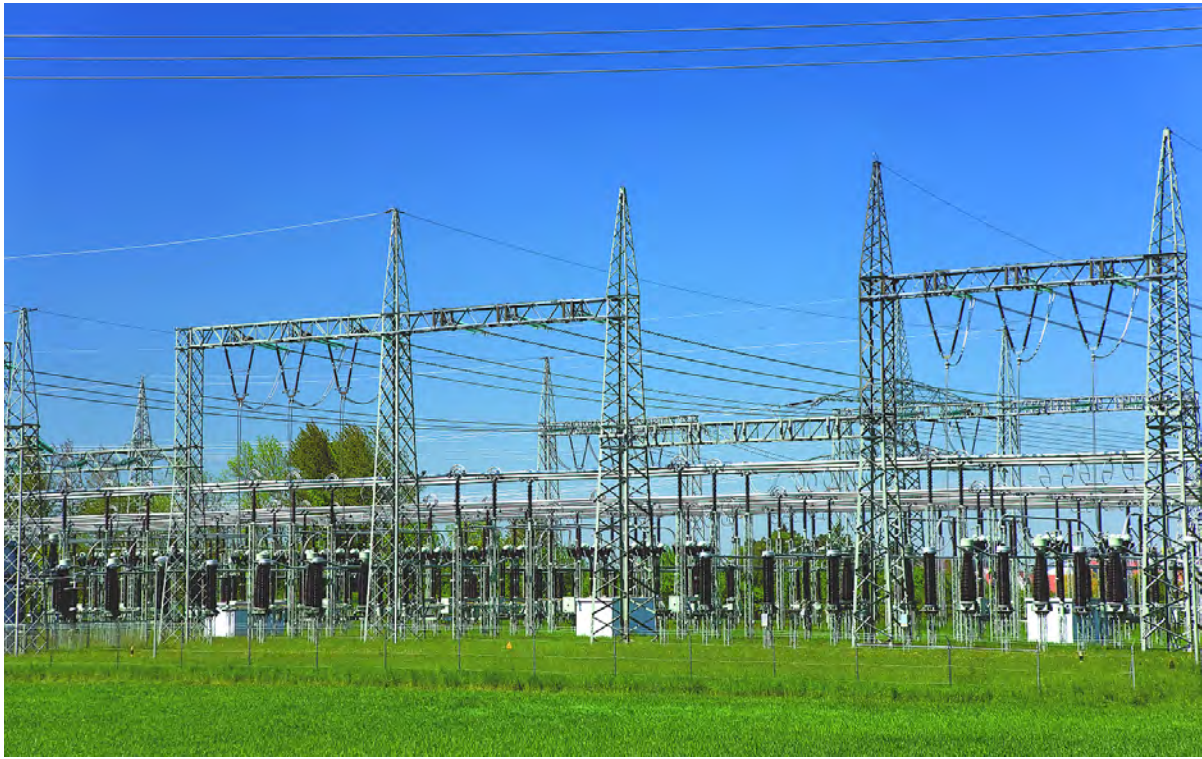
Figure 3: Outdoor switchgear with hollow tubular conductors and overhead lines
